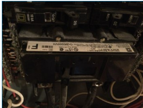
200 amp in main panel
