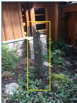
Remove decayed stump left of main entrance, where heavy WDC insect activity is noted.
