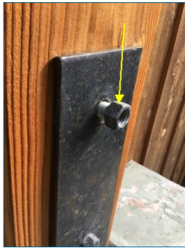
Several nuts are loose at post brackets, have technician lock-tight and seat all nuts.
