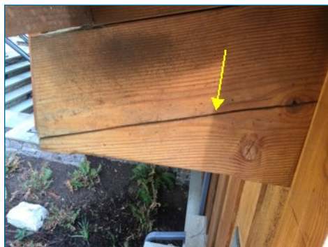
Larger splits in extruded lumber tails, prep and seal with chinking putty or preserve.
