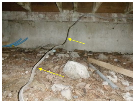
Surface mounted wiring noted under deck, electrical should have been ran in conduit to reduce risk of physical damaged
