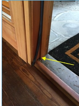
Weather stripping failing at front door, replace/repair.
