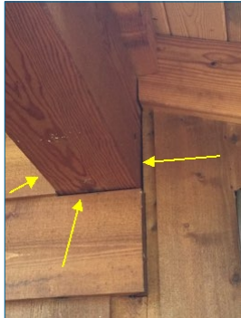
Caulk/seal siding at stone wall connection, where weather barrier is exposed.
