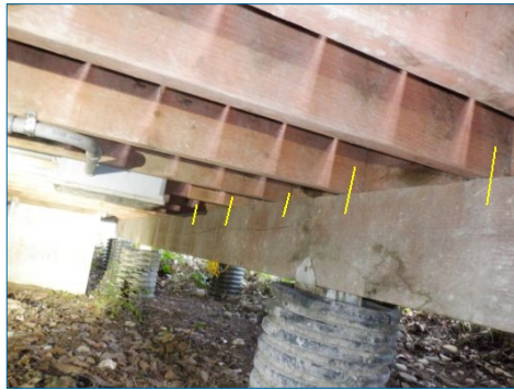
Beam and joist connections were missing strapping/hurricane clips (H1 clips). Have required strapping installed to bring up to current regional building requirements.
