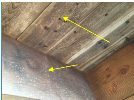
Organic growth in eaves, treat/clean and seal during routine maintenance.
