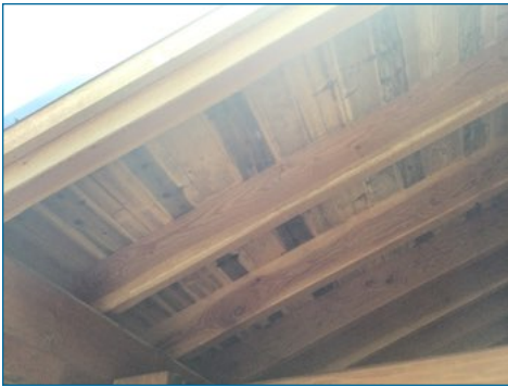
Organic growth in eaves, treat/clean and seal during routine maintenance. Note dark sporing in entry eave.
