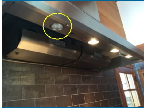
Left bulb burnt out, replace.
