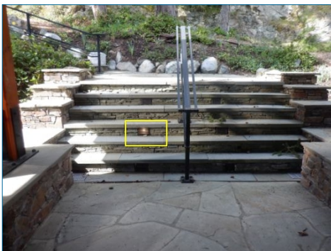
Single step light lit when operated then went out, have light checked for serviceability.
