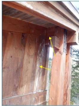
Bird nesting noted in various areas of eaves, Clean bird waste and screen off points of access to prevent unwarranted damage to structure.
