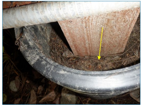
Post under deck have form tube around post, recommend removing black plastic forms to prevent debris and water from being held against wood post, promoting premature decay.
