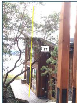
Tree limbs within 10 feet of roof should be trimmed away to provide air and sunlight to roof, while minimizing debris & dampness. Trim back tree on east side of structure.
