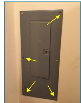
Panel cover missing screws, install where missing to better secure. ( X6 )
