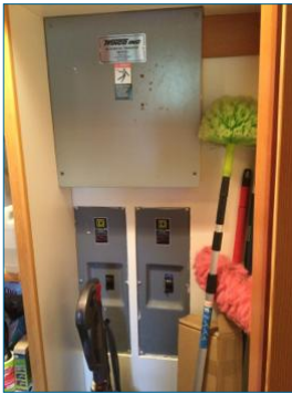
Generator auto switch located in hall closet.
