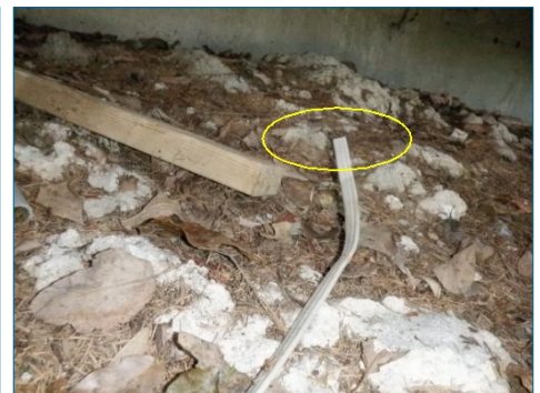
Electrical line under deck not properly terminated, have line capped and terminated in junction box.
